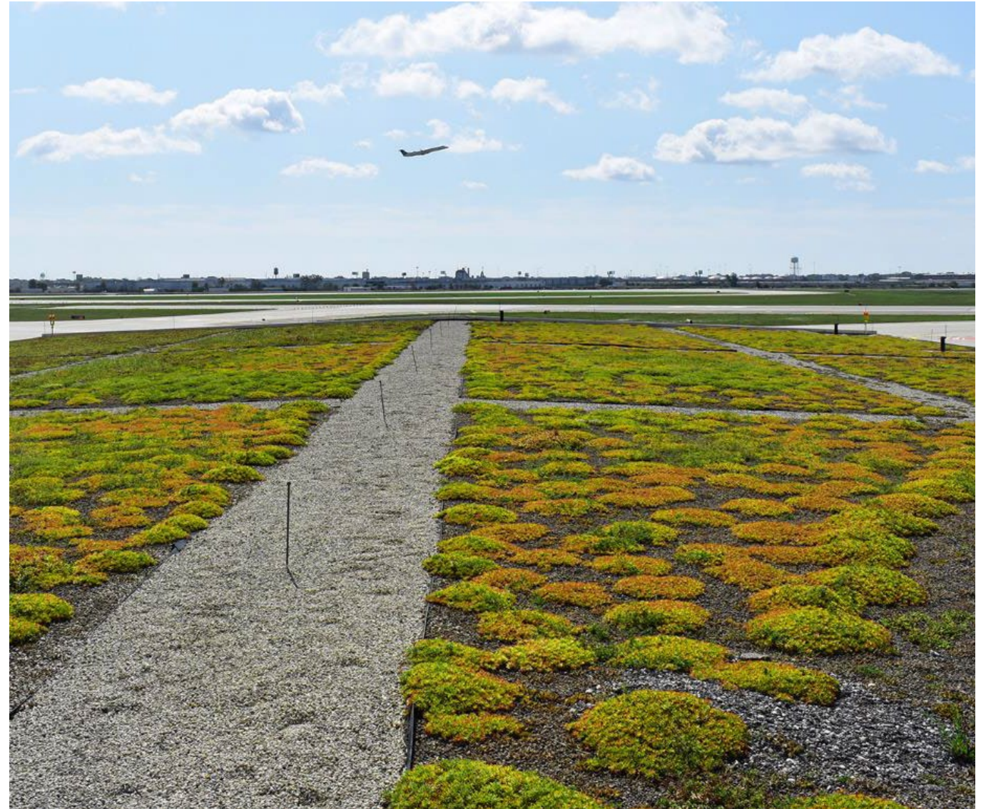
ORD Lighting Control Vault Green Roof
